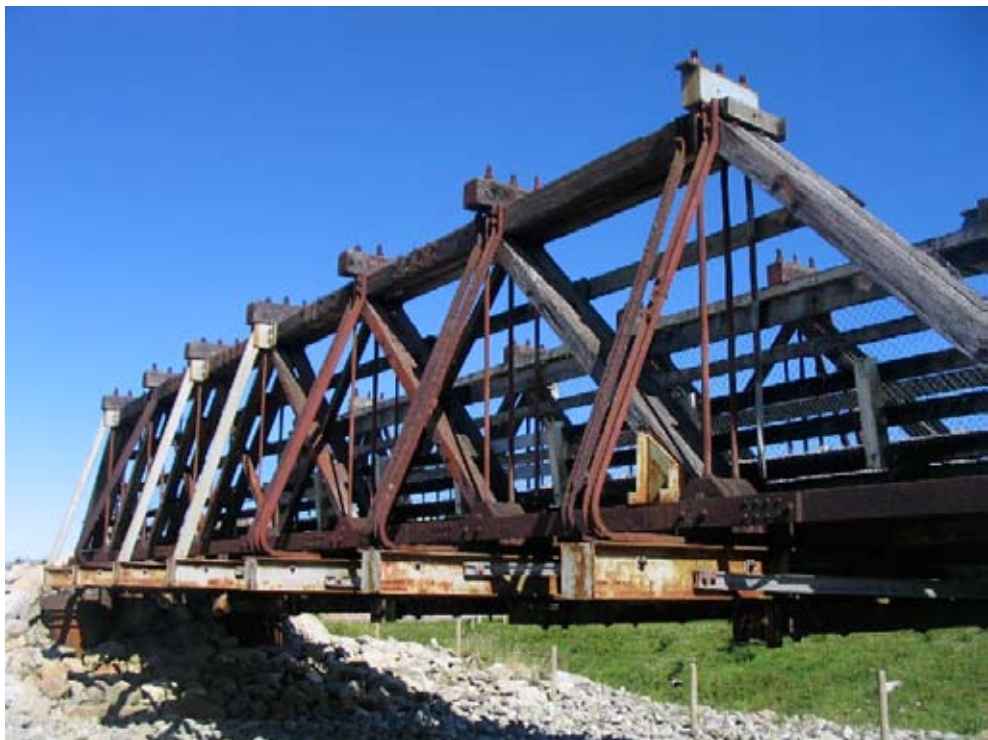
A section of the historic road and rail bridge over the Arahura River has been preserved.
